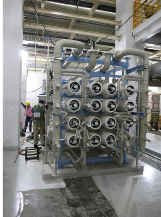
Reverse Osmoses Skid
